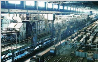
Horizontal furnace for continuous galvanizing line
